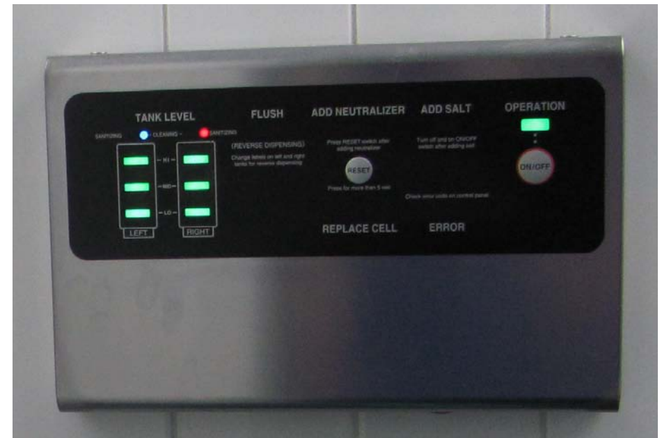
EWATER REMOTE CONTROL UNIT
